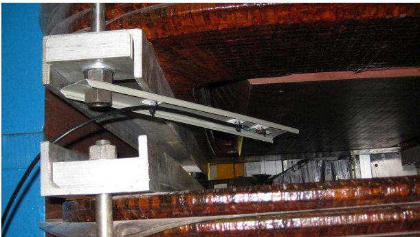
Figure 2: POMPOM #2 installed in D2. The sensor PCB itself is the white chip to the right of the final cable-tie.
